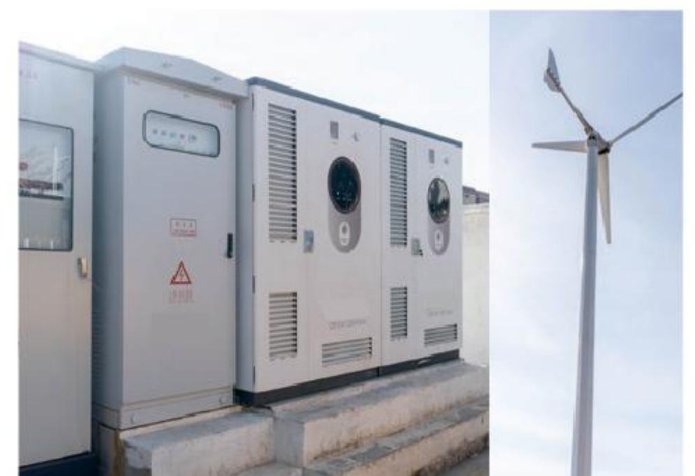
250KW/522KWH in Mespal Head quarters project
