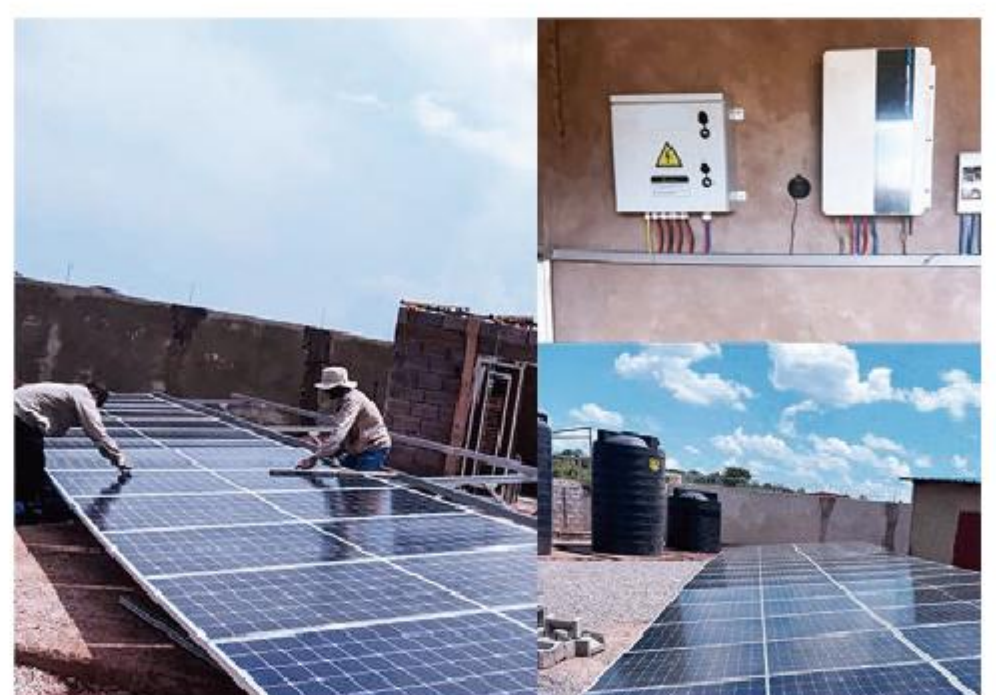
30KW off-grid solar system in DR
