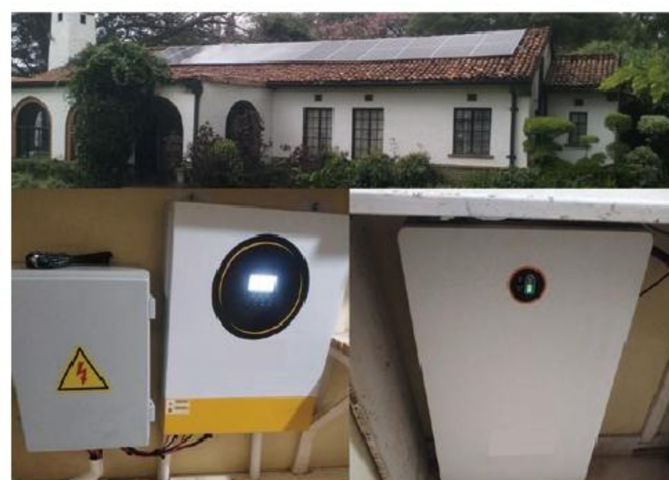
6.6KWP solar+8.5KW/10.24KWH offgrid solar system in Kenya
