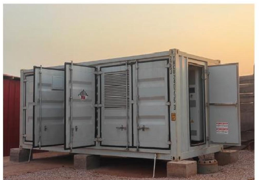
500KW+1MWH BESS project in Tan
