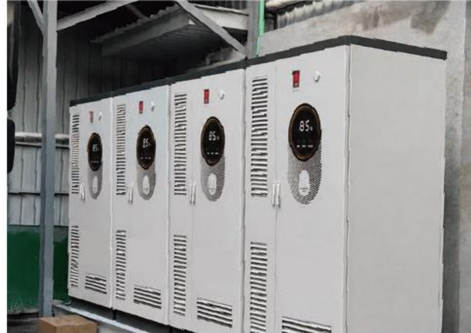
0.46MW/0.916MWH in Huzhou Siyi factory
