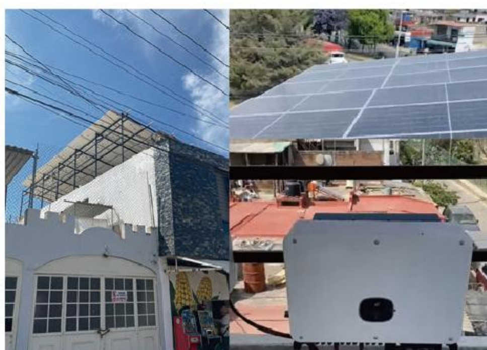
20KW on-grid solar system in Mexico
