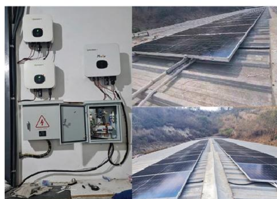
22KW on-grid solar system in Ecuador
