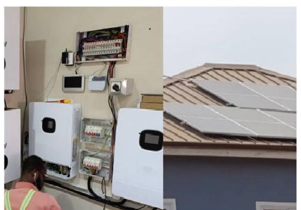
8KW solar+ 20KW/20KWH Off-Grid System in Accra, Ghana
