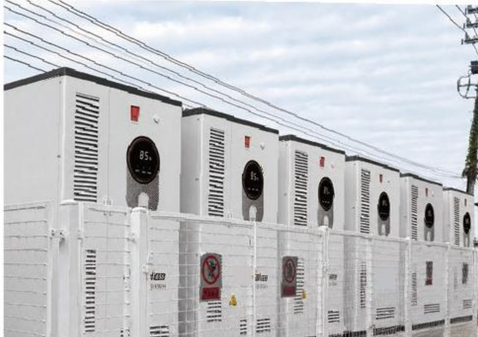
0.92MW/1.832MWH in Huzhou Tianlin Textile factory
